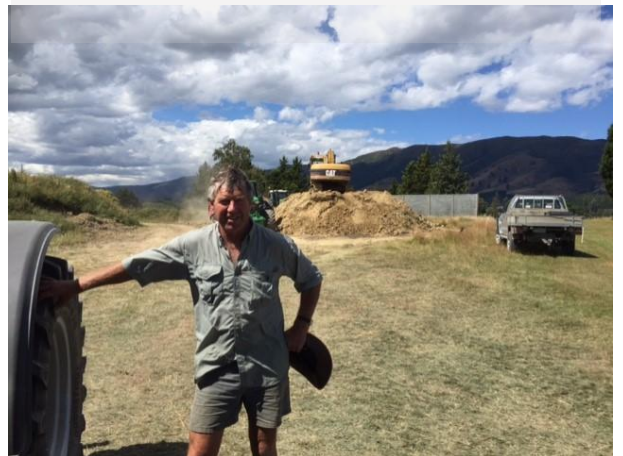
Lions assisted with the relocation of superfluous dirt from the site of the Ribbonwood Rest home Extension
