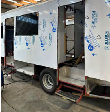
Side of Vehicle as at November with 55inch TV in place.
