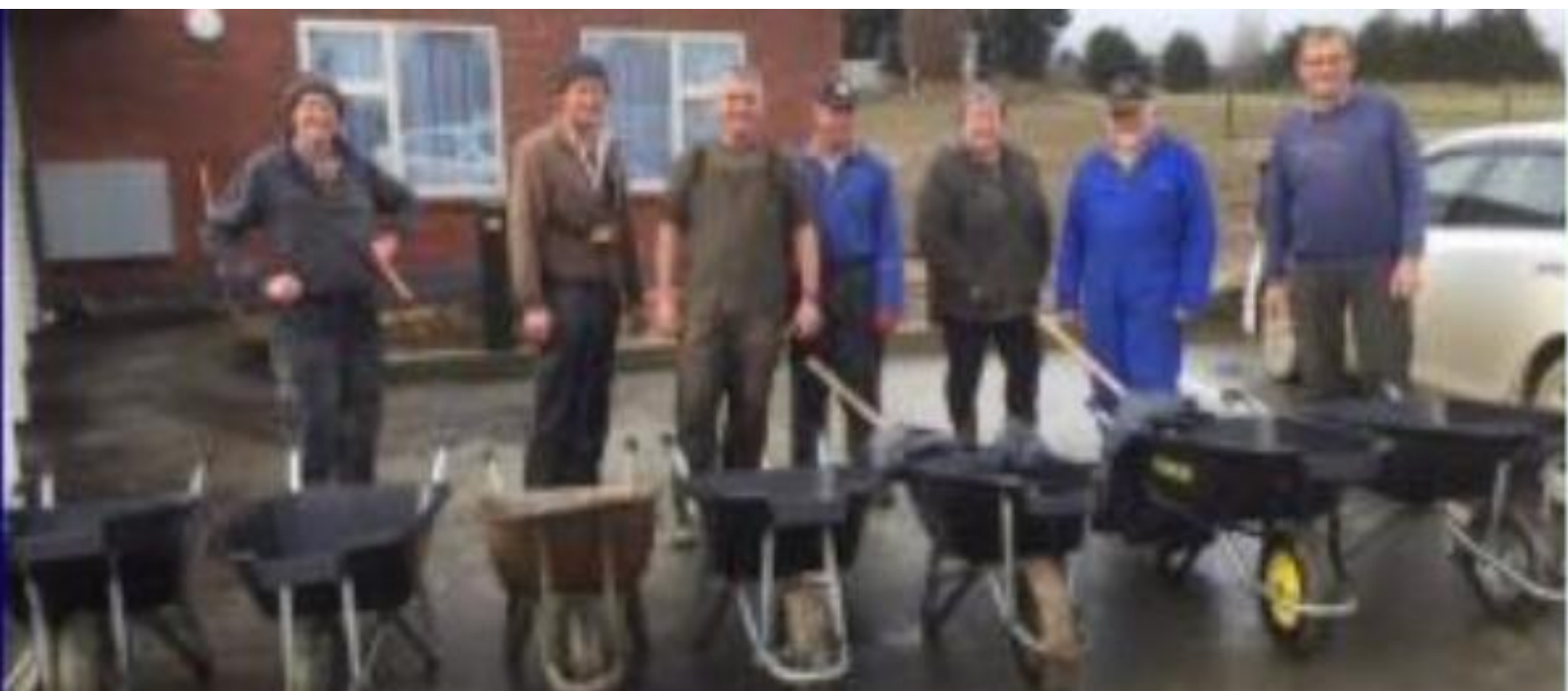
West Otago Lions team concreting at the West Otago Rest home extension ↓
