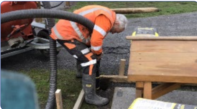
Kaikoura Lions - building 3 more canopies for picnic tables. A sucking hole machine is easier than digging, driving or ... then poles slip in.
